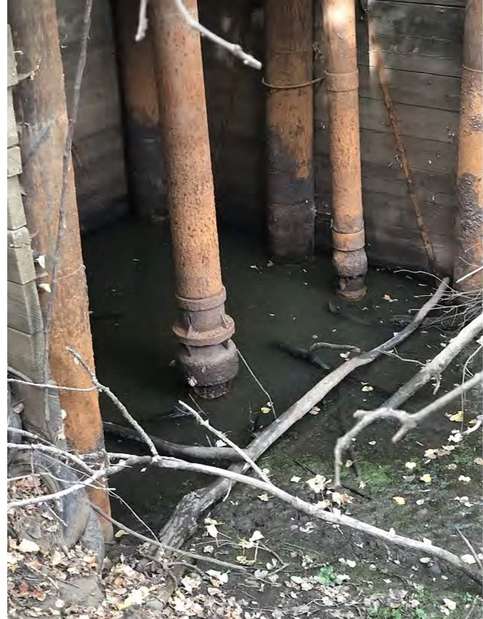
EXISTING PUMP BOWLS AT INTAKE CHANNEL
