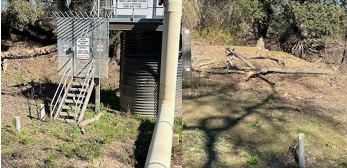
Fallen Limb Near Pump Station
