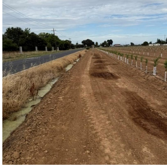
New Leaks along Brandt Road stretch half way to the outfall
