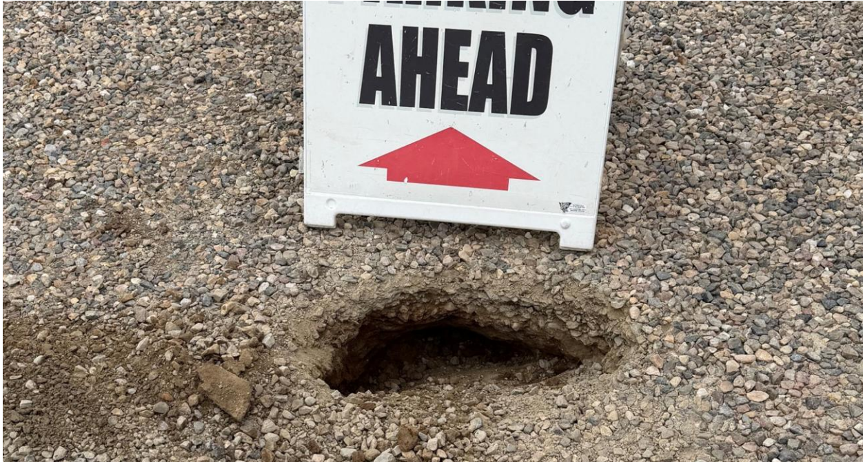
Staff filled this Harney Lane Pothole two weekends ago and Arnaud did a permanent repair last week
