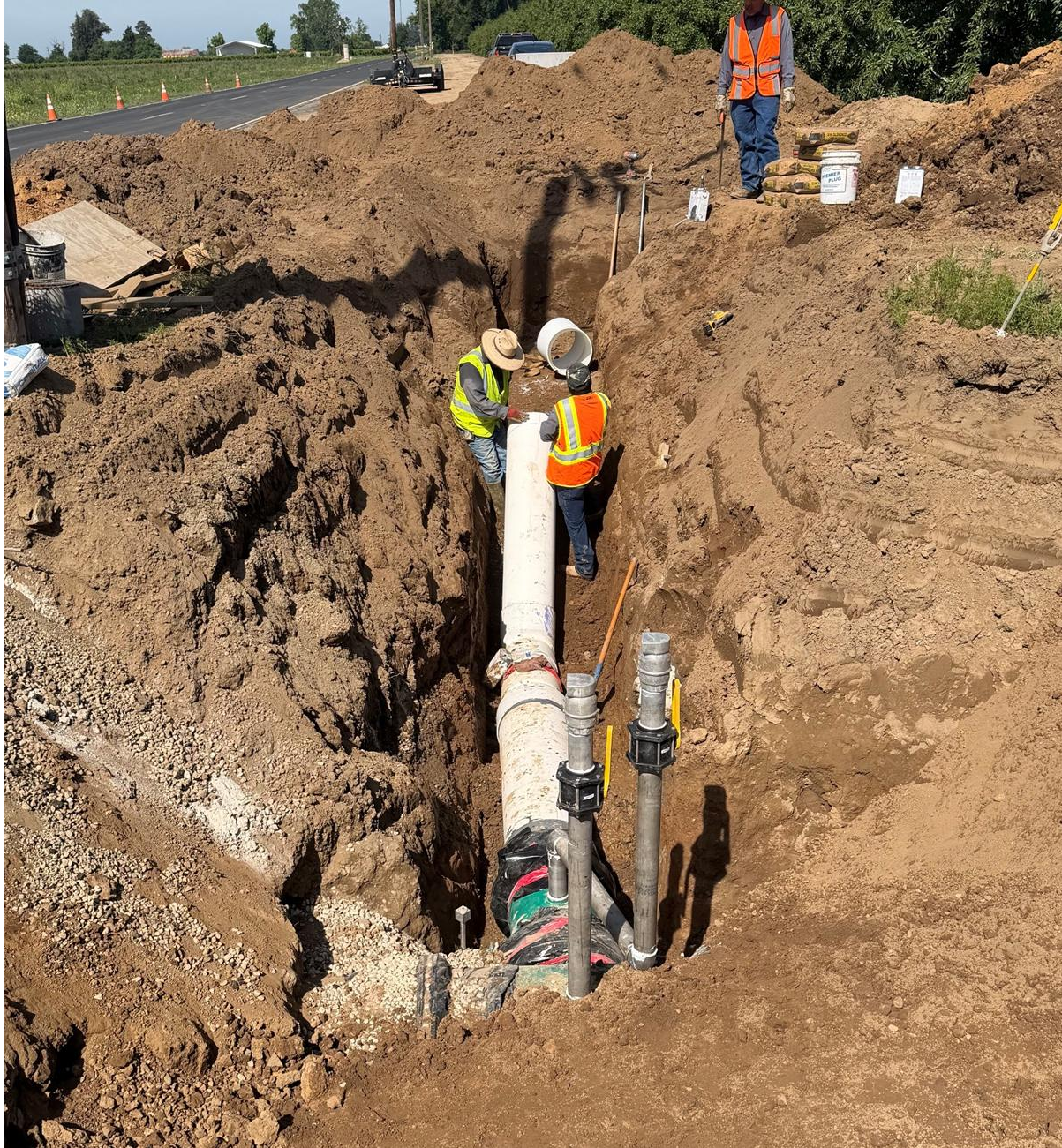
Creekside's SWEEP Grant irrigation contractor installs the private connection to the North Sytem Main after the final 42 inch line was connected.
