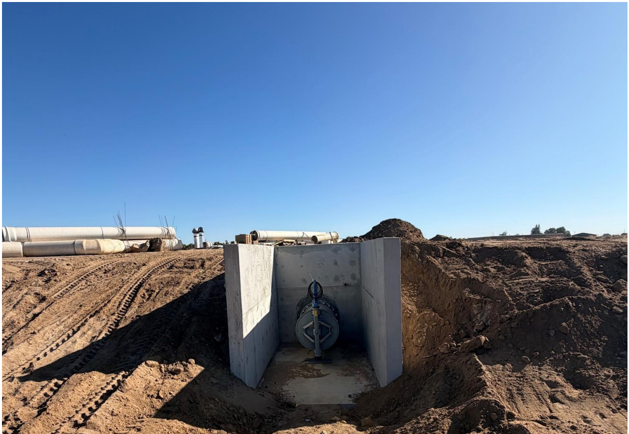
The New Rubicon automated valves and meters are installed at Teck Basin
